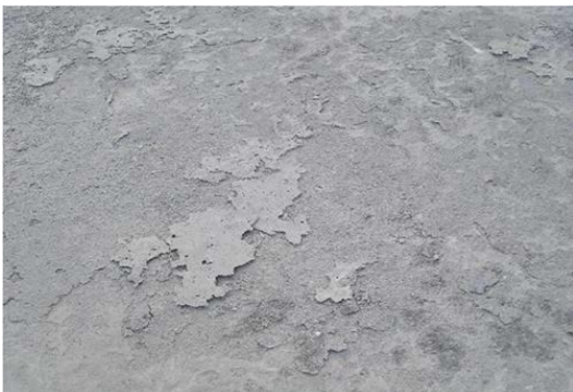
Figure 3 – example of surface laitance
