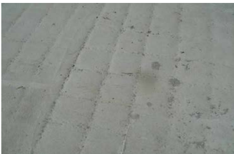
Figure 2 – example of 'reinforcement ripple'
